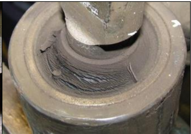
Figure 5-3; Acceptable surface cracks
